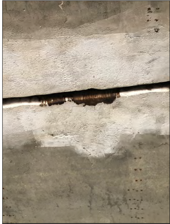
Picture 6—Guano stains at ceiling joint; 17 SEP 2020.
