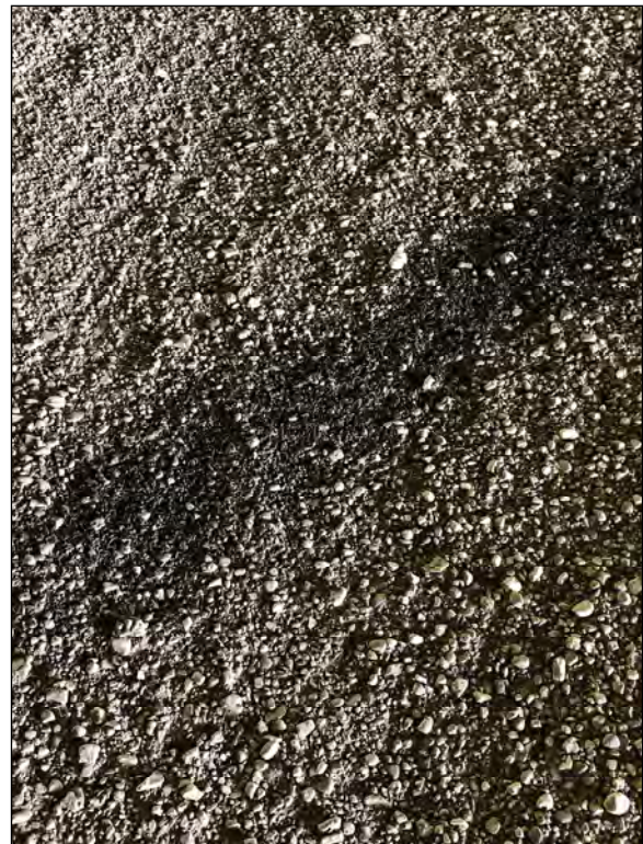
Picture 4—Center span guano pile; 17 SEP 2020.
