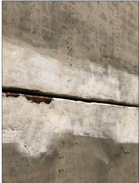
Picture 8—Ceiling joint; 17 Sep 2020.
