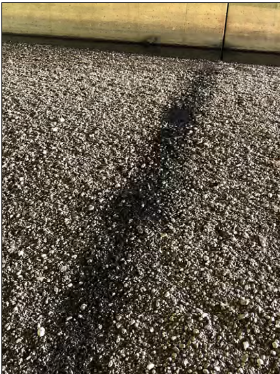
Picture 3—Center span guano pile; 17 SEP 2020.
