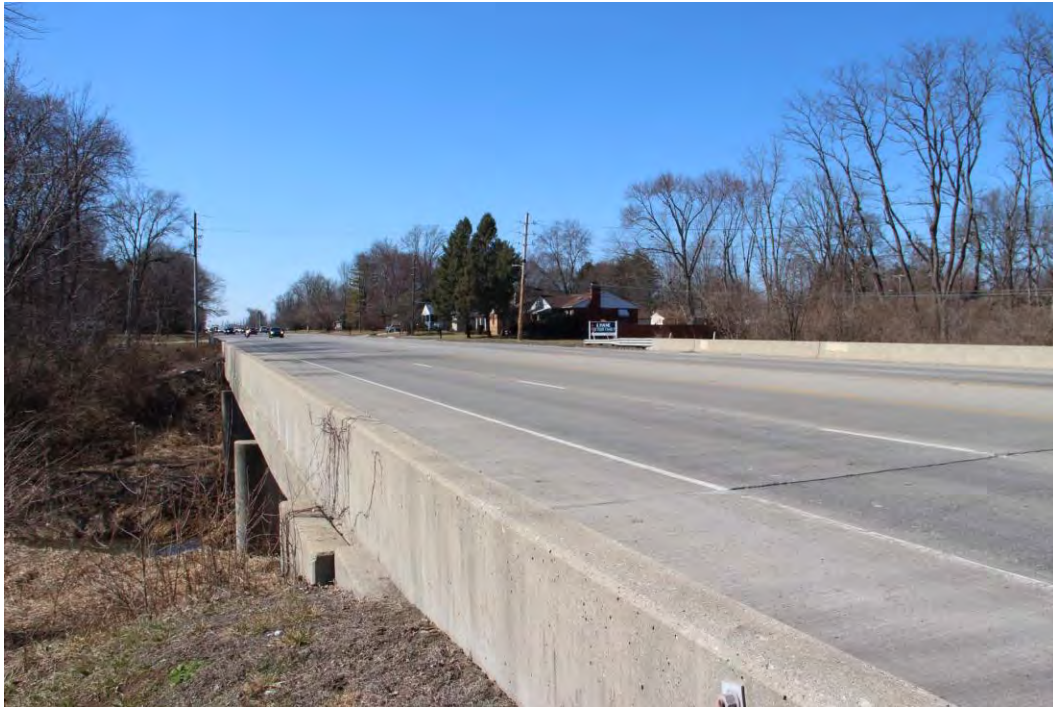
Photo D-21. MB-035, bridge carrying US 36 over the Little White Lick Creek showing the south approach, facing west.
