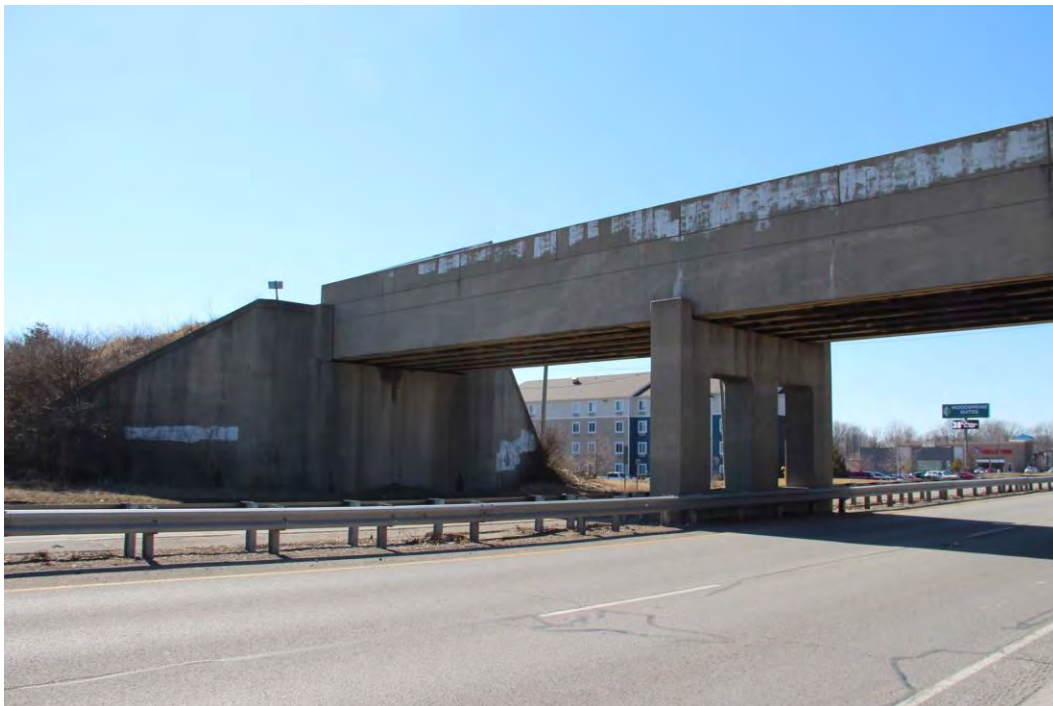
Photo D-26. MB-036, east elevation of bridge carrying railroad tracks over US 36 showing center pier and south abutment, facing southwest.
