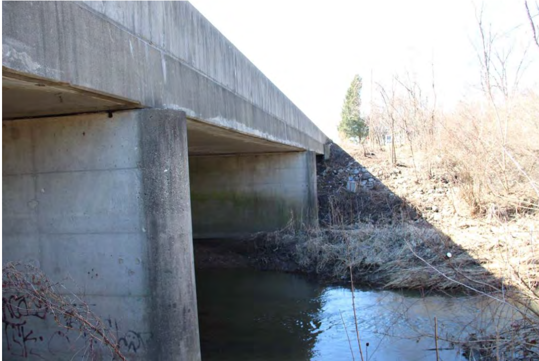
Photo D-19. MB-035, bridge carrying US 36 over the Little White Lick Creek showing the south elevation, facing northeast.
