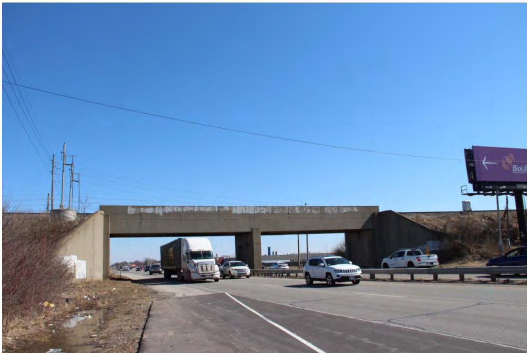
Photo D-24. MB-036, bridge carrying railroad tracks over US 36 showing the west elevation, facing east.
