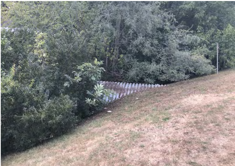
Photo 47 - Shiloh Creek Culvert, Southwest View, (Map 2) -17 SEP 2020
