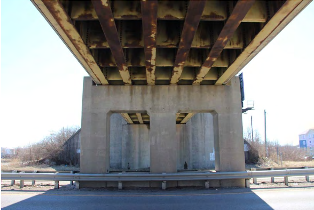
Photo D-25. MB-036, bridge carrying railroad tracks over US 36 showing center pier, floor beams, and south abutment, facing south.
