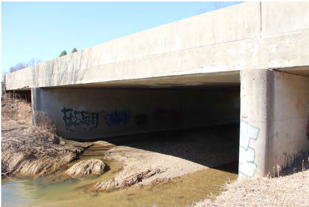
Photo D-20. MB-035, bridge carrying US 36 over the Little White Lick Creek showing the north elevation, facing southeast.
