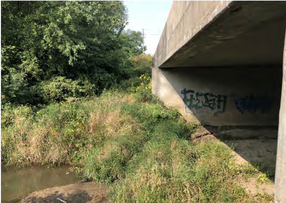
Photo 137- East Fork White Lick Creek Bridge Southwest Corner, West View, (Map 5) - 17 SEP 2020
