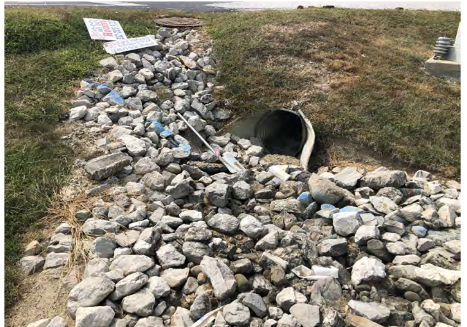
Photo 148 - US 36 and Country Club Road Northeast Corner Drainage West View, (Map 6) - 17 SEP 2020
