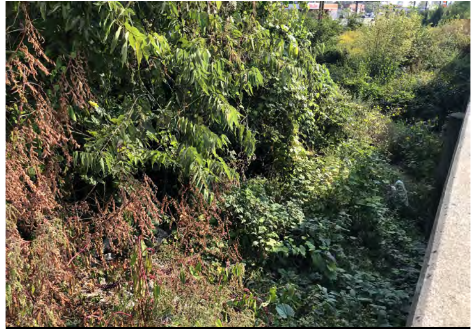
Photo 138- East Fork White Lick Creek Bridge Northwest Corner, Northeast View, (Map 5) - 17 SEP 2020
