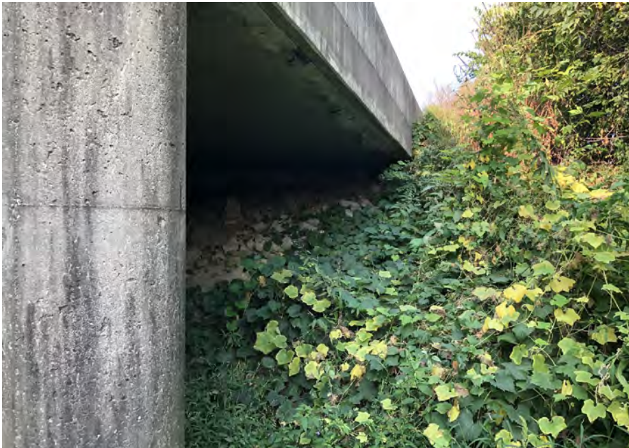
Photo 139- East Fork White Lick Creek Bridge Northwest Corner, West View, (Map 5) - 17 SEP 2020
